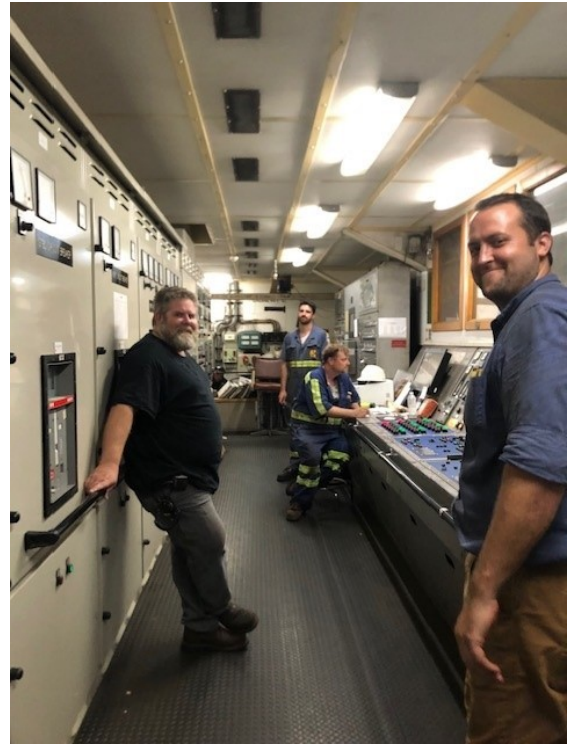
Licensed engine officers in the Edmont's Engine Control Room
